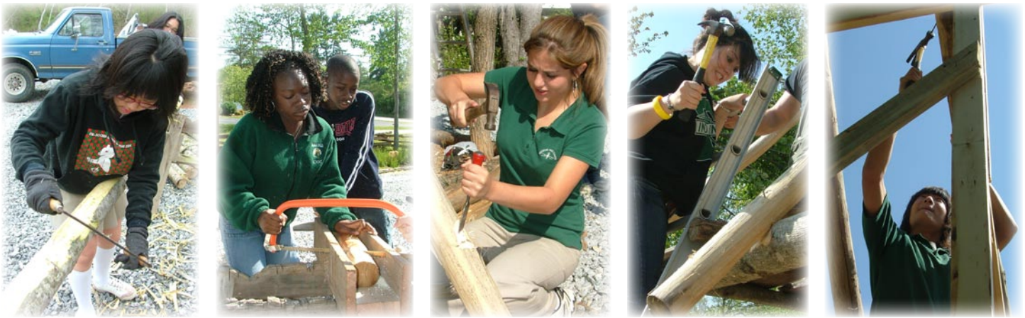
Above are students performing each part of the process of making and installing a rafter on the Nicholson Cabin: skinning bark from the poplar logs, sawing the angled top end, notching the lower end, and nailing bottom and top ends in place on the cabin.
